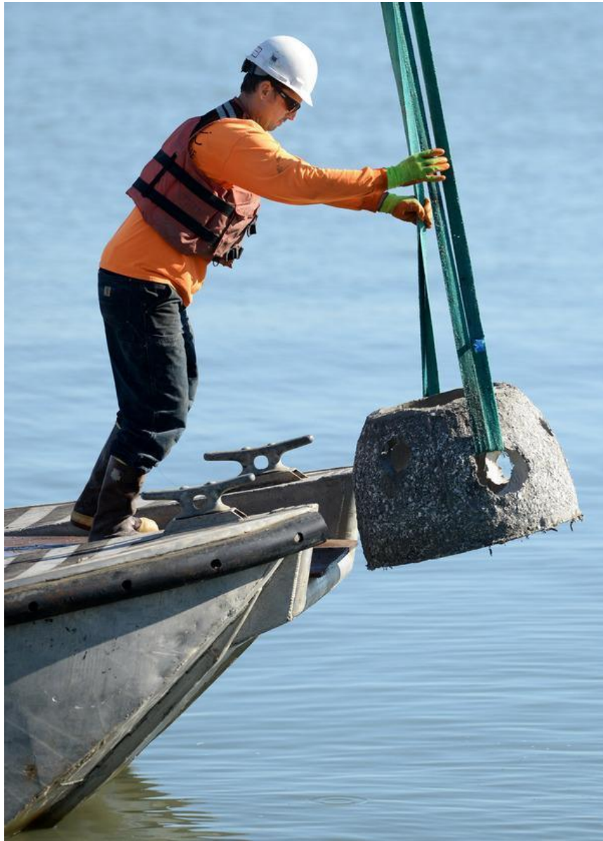
Ethan Livingston, of Dixon Marine Services, lowers an oyster reef ball into San Pablo Bay off Point Pinole Regional Shoreline in Richmond, Calif., on Friday, Nov. 15, 2013. The Watershed Project is installing 100 of the man-made "balls" to promote the establishment of plant and animal life in the area. Dixon Marine donated their services. (Dan Honda/Bay Area News Group)
